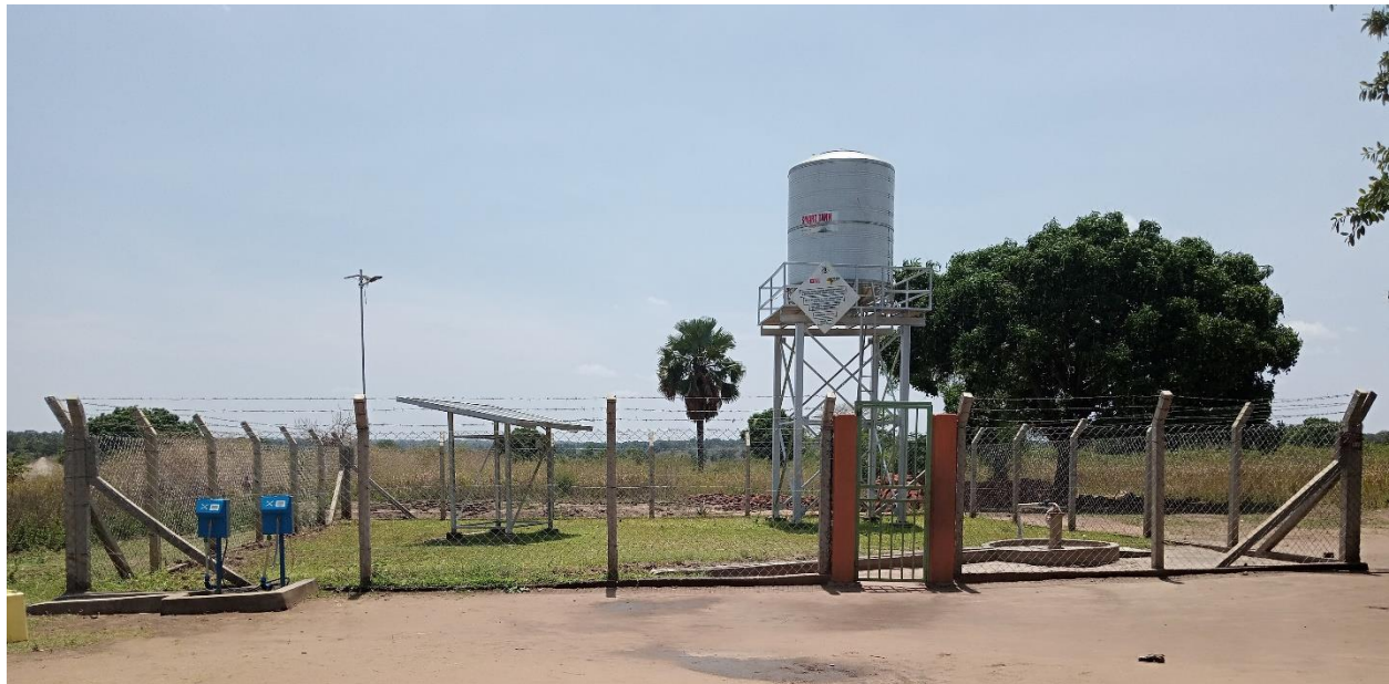
Photo: Mini Solar Powered Water Supply Systems at Zinjo Constructed by ACORD Uganda in Bidi Bidi Settlement
